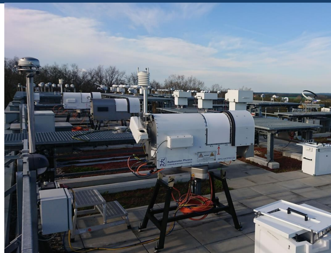
Fig.1: HATPROs on the roof of the DWD.
